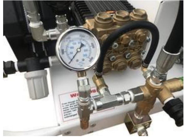
Figure #26 – Pressure Gauge / Manometer
