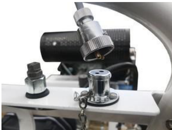
Figure #17 – Feed Pump Connection
